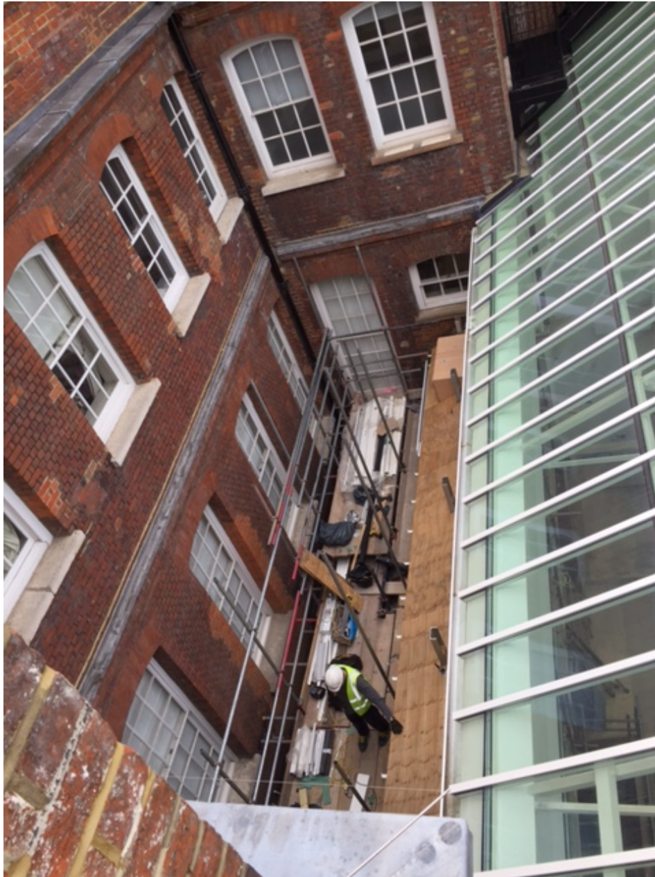
Atrium roof of 11 Floral Street adjacent to 43 King Street (Works taking place to refurbish atrium glazing in connection with permitted works on site)
